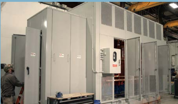
UNIClad transformer in Roanoke
